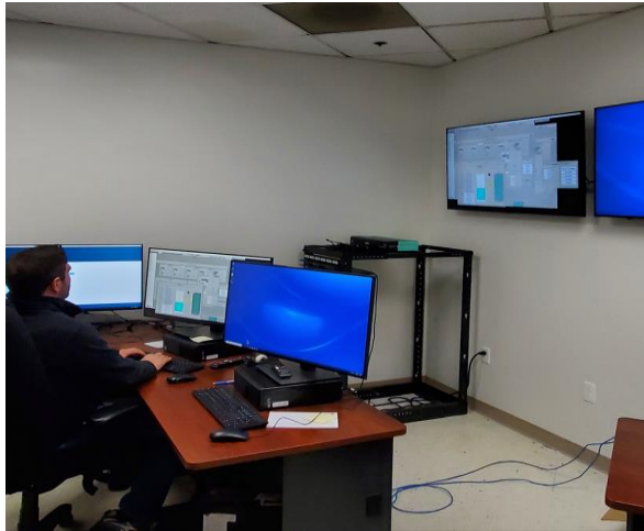
Supervisory Control and Data Acquisition System (SCADA) Installation at Ettie Street Pump Station
